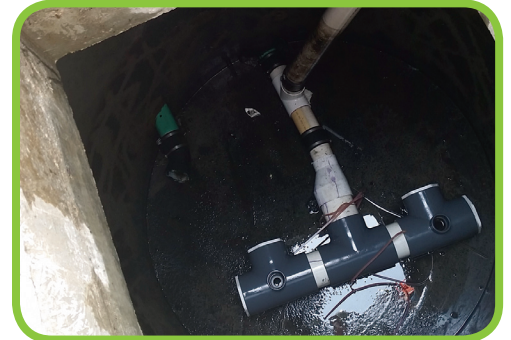
Manifold Tee View of a Cleaned System
